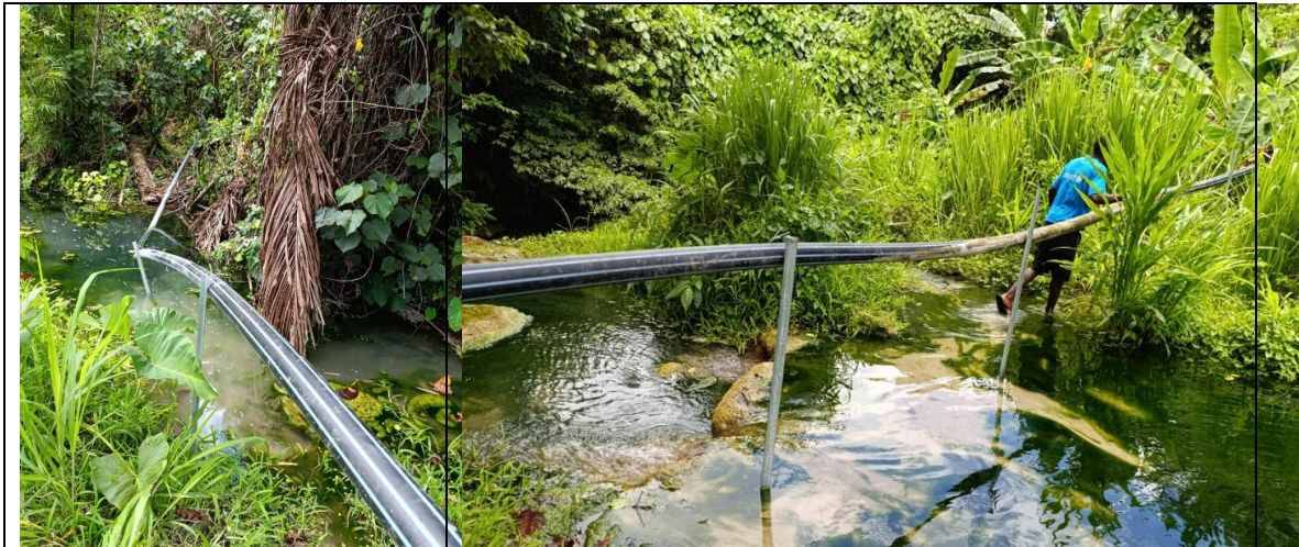
Photo #1; the first water section (the photo is taken from the 2 nd pier location, looking toward the 1 st pier) Photo #2; the second water crossing- right side is the anticipated the 3 rd pier.
